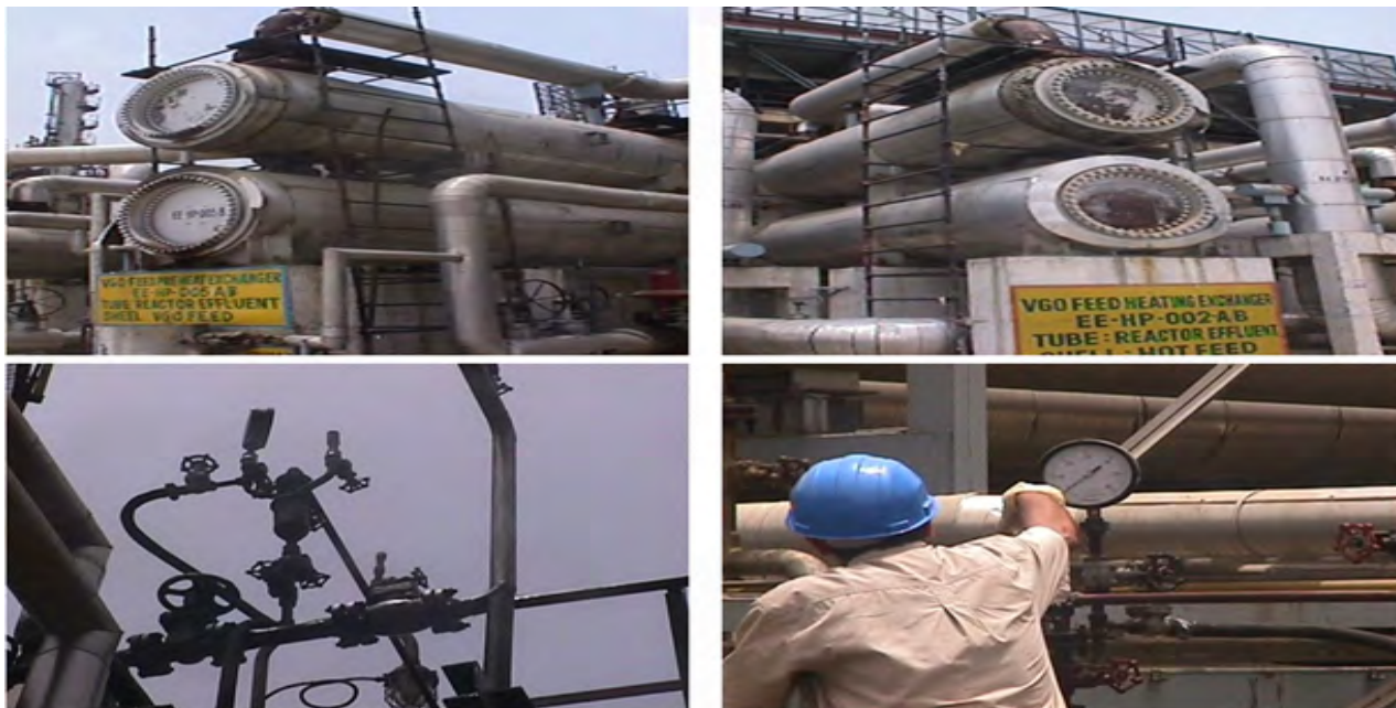
Radiotracers for Leak Detection in Heat Exchangers
