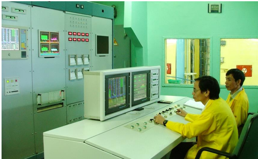
Fig. 3. Main console in the control room of DNRR
