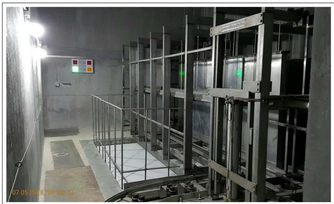
Fig. 5: The moving subsystem of VINAGA1 at the Danang irradiation center
