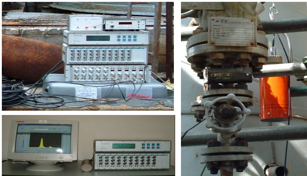
Fig. 7: The Tracer Data Acquisition System 10 channels TDAS (left)- detector installed in pipe line (right)
