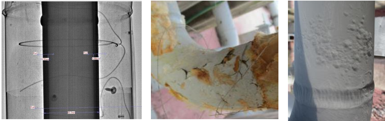
Figure 3. CUI location detected by DR (before and after surface treatment)
